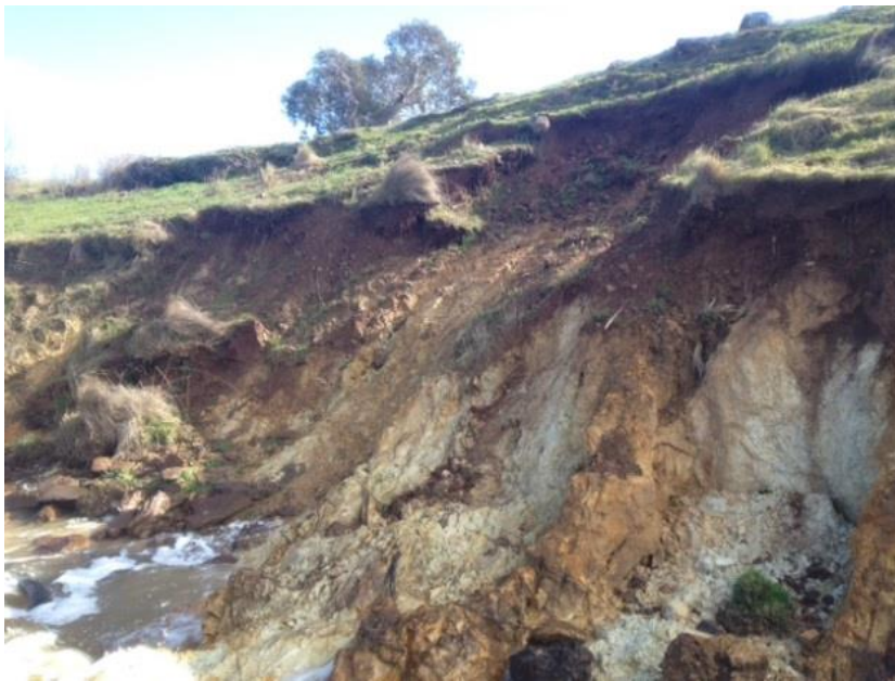
Figure 9: Foreshore erosion and landslip at Upper Coliban Reservoir in 2013
