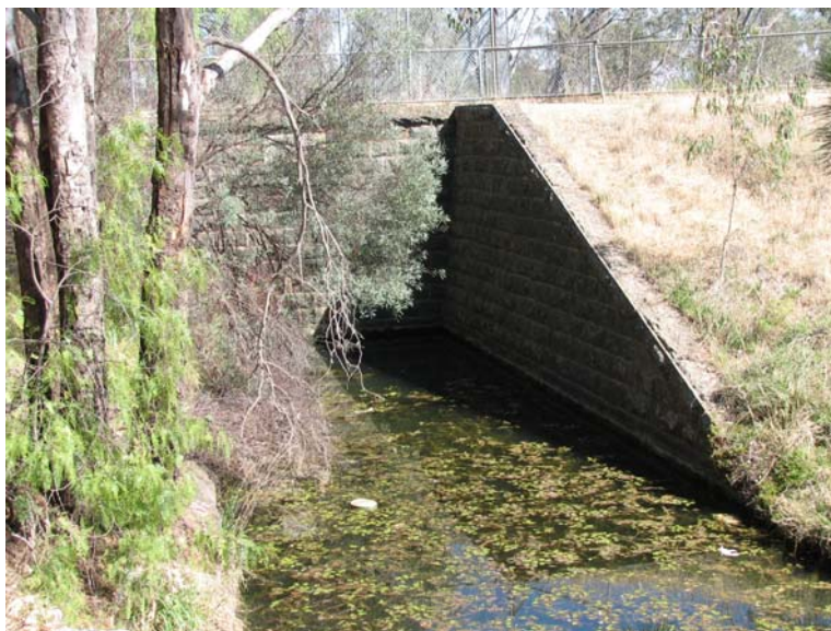
Loddon United Waterworks Trust Headworks at Bridgewater on the Loddon River built 1884.
