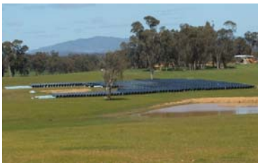
All of the Stage 2a and 2b pipes have been delivered to storage yards along the pipeline route and in Bendigo
