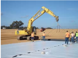
Lining of brine lagoons at Bendigo Recycled Water Factory earlier this month.
