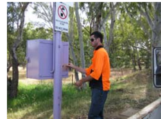
Customer obtaining water at Stanley Street Standpipe
