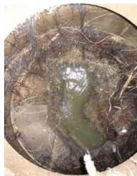
Above: Tree roots in the sewerage system
