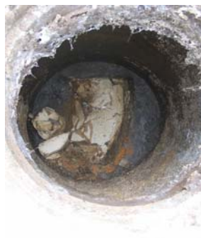
Above: Fat in the sewerage system
