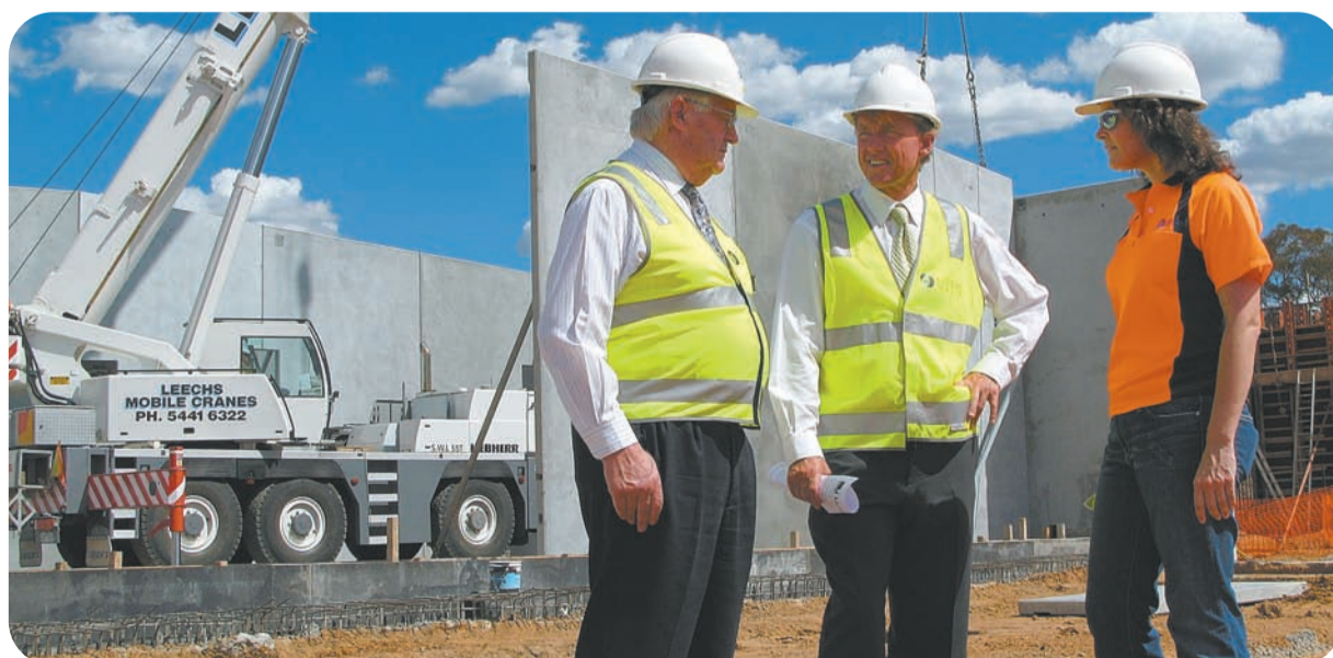
Chairman Gordon McKern, Minister for Water John Thwaites, and BECA Project Manager Anthea Ross on site this week at the Recycled Water Factory at Bendigo Water Reclamation Plant.
