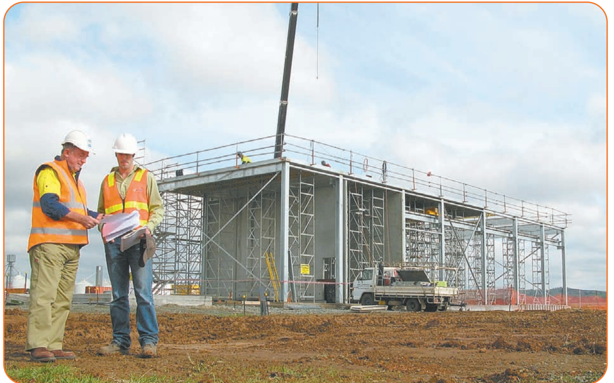
Above: Kevin McGlenn, Compliance and Design Manager and John McNamara, Site Engineer at the pump station site in Colbinabbin.
